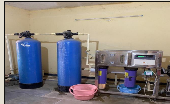
RO plant in Gram Panchayat office
