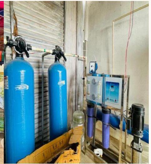
RO Water Plant
