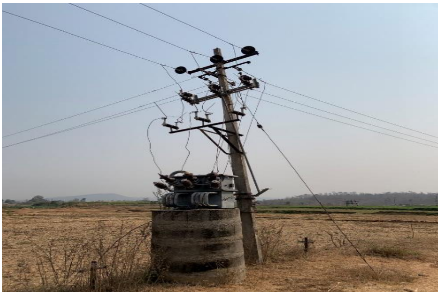
Photo: Electricity Tower in the village.
