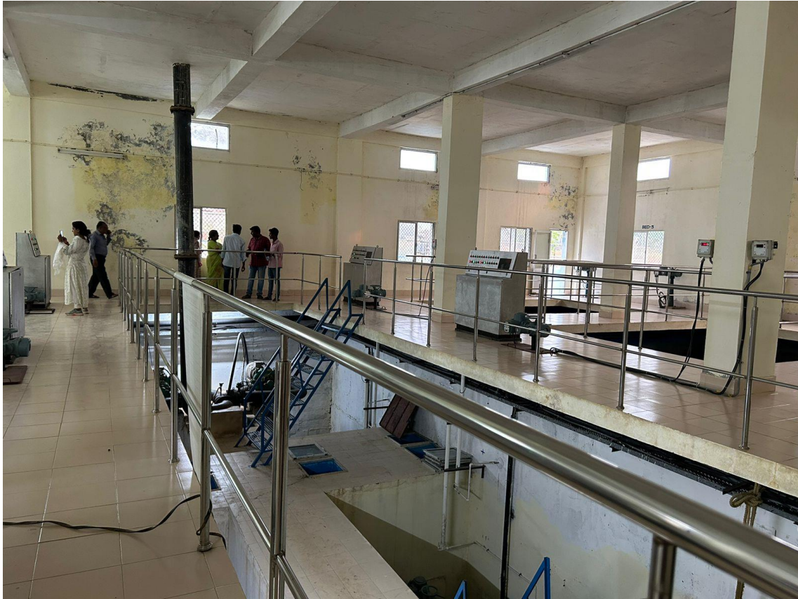
Photo: Water Treatment Plant under Mission Bhageeratha.
