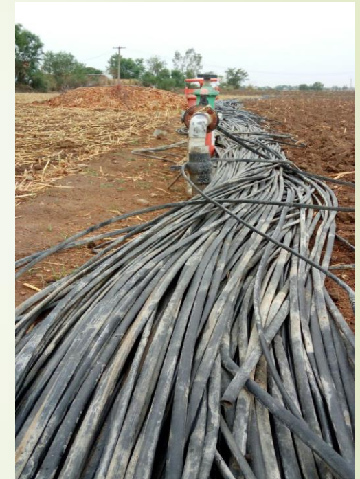
Drip irrigation Pump and Pipes in village field
