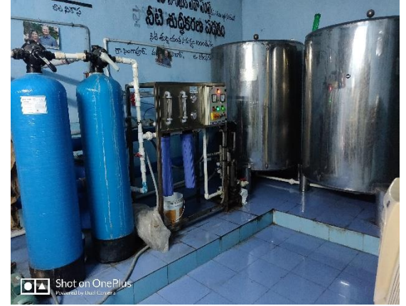
Water Purification Plant
