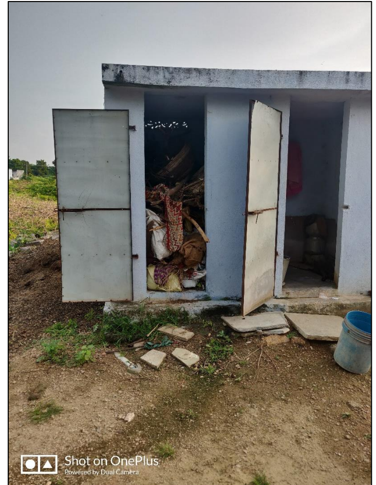
Toilet being utilized for other Purposes
