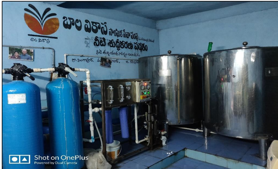
BALA VIKASA Water Purification Plant
