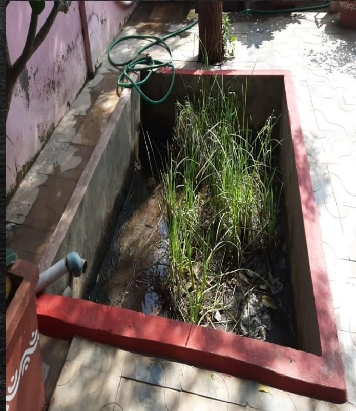
Soak pit and Rain water harvester
